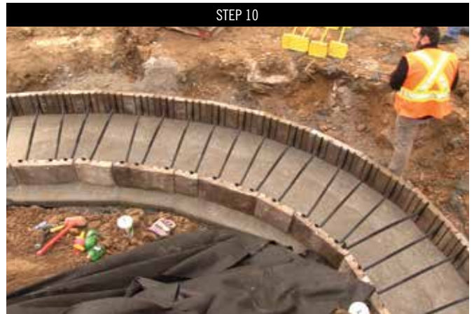
Laying out the radii. Insert plastic connecting members into the veneer dovetails to keep the connectors as straight as possible. Make sure that each veneer has at least two connecting members for proper panel support.
