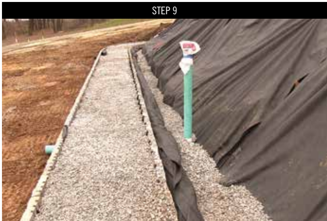
Place the drain tile directly behind the rear wall panel to provide for positive drainage through the wall to daylight.
